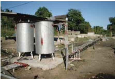
Biogas powered electric power generator: Collected biogas can be used as fuel to power electric generators (as shown above) or for direct use in cooking, lighting or heating.
